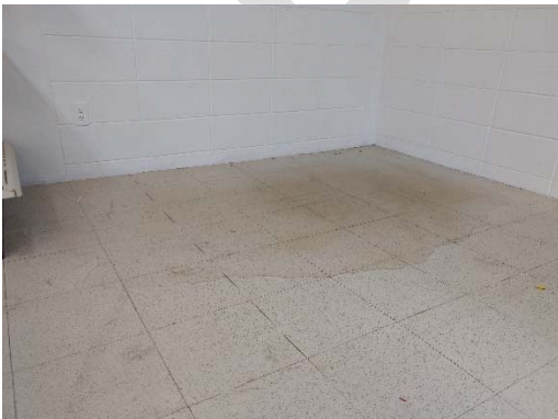
WATER ON FLOOR BUT WALL IS DRY
