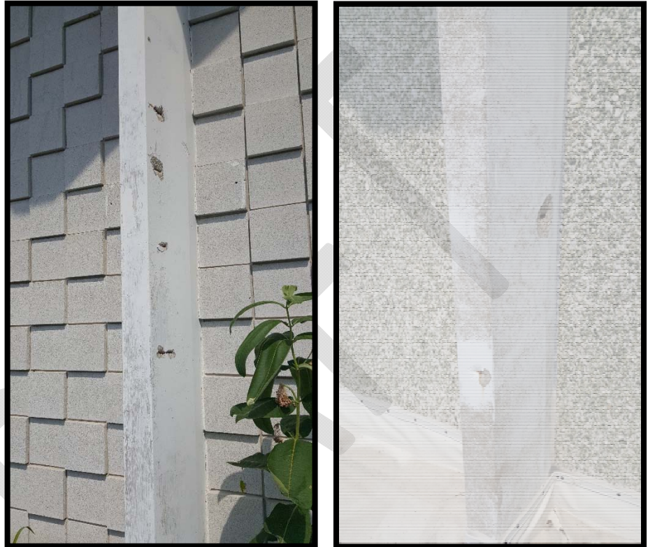
Figure 1 : columns spalled concrete exposing re-bar
